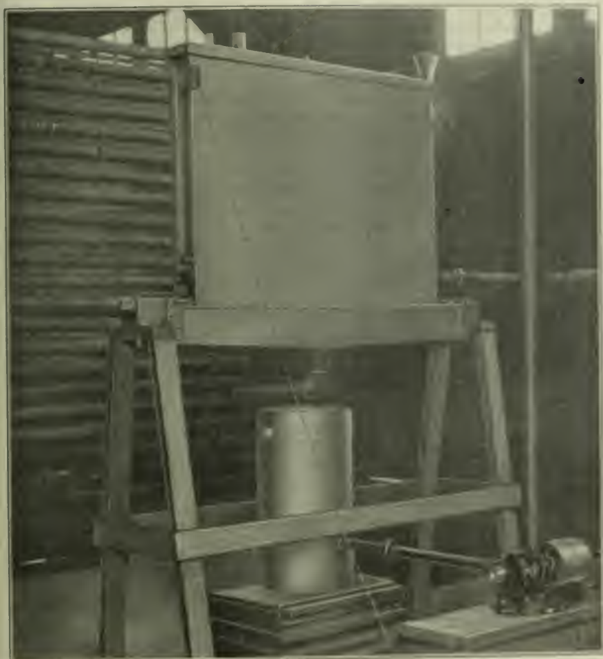
FIG. 3. AN ICE PLANT INSTALLATION OF THE PENNELL CONDENSER
